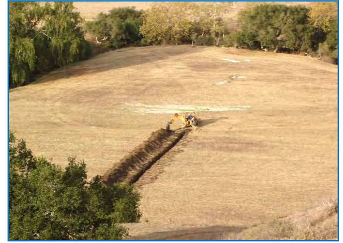
Figure 78. Backhoe used to install pipe in hayfield in order to get 48" depth.
