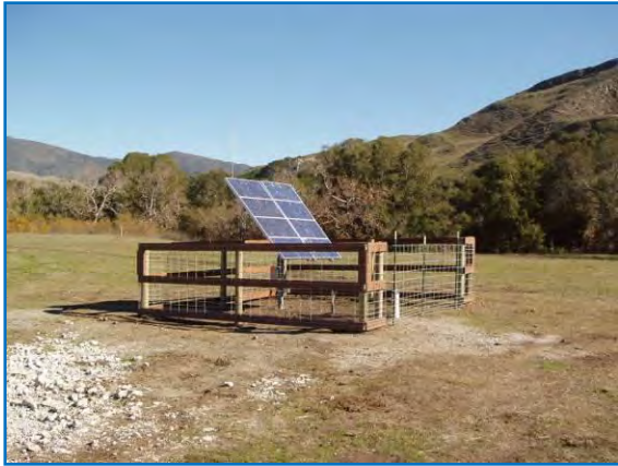
Figure 82. Solar panel and pump manifold at well site #2.
