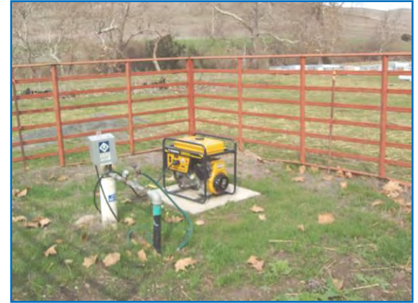
Figure 10. Well and generator.
