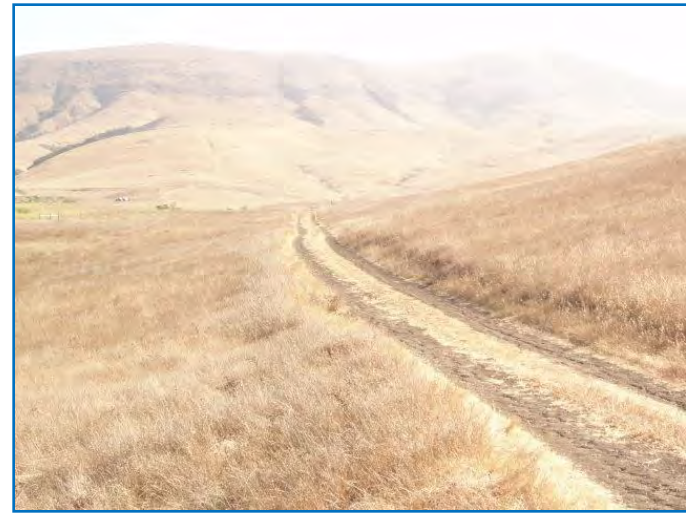
Figure 65. Rilling evident on unvegetated portions of road.
