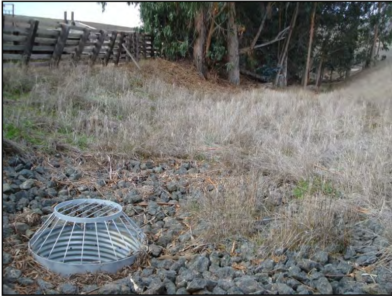
Figure 25a. Looking upstream at drop structure and restored headcut, over a year after installation
