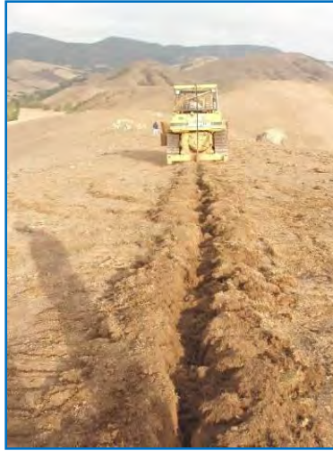
Figure 77. Ripping in pipe.
