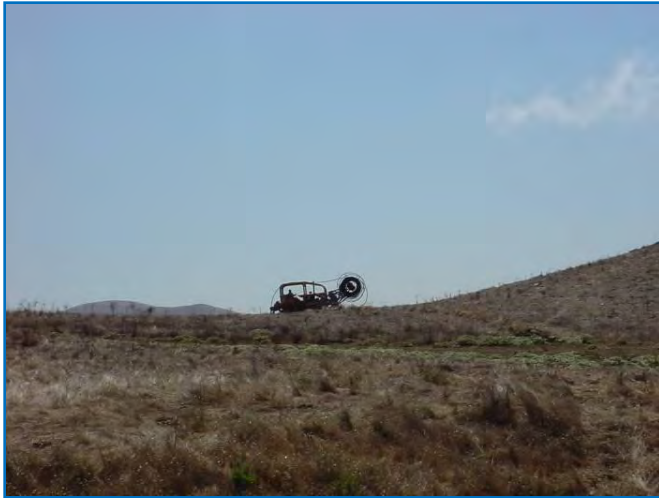
Figure 6. Distant view of cat ripping in pipe – note spool of pipe on right side of cat.
