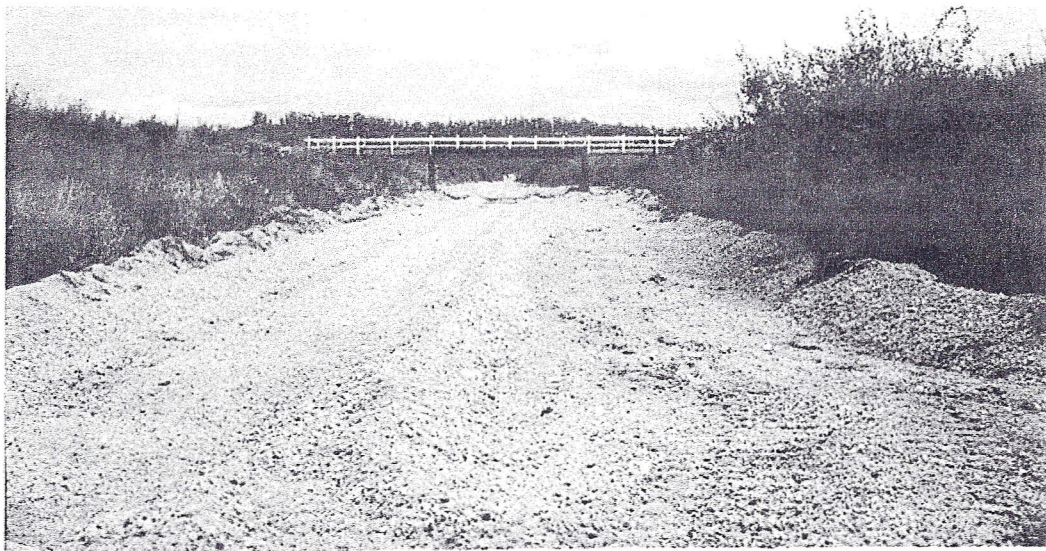
Looking up stream at county road bridge from S.P.R.R. bridge showing channel conditions. 10/29/56
