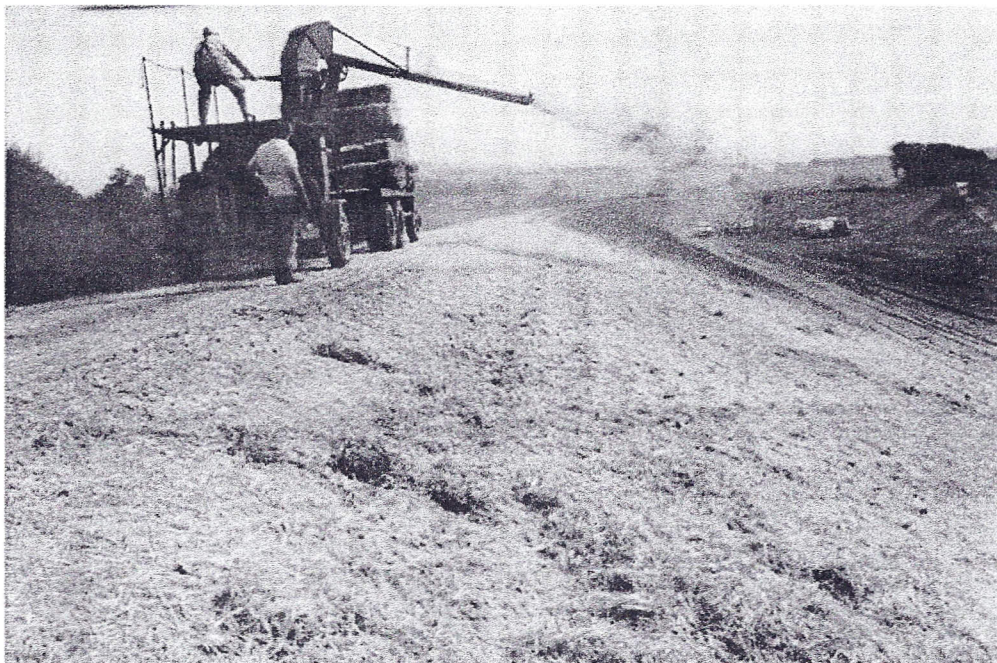
AG SCD PL 566 -Straw blowing machine placing straw on side slopes of dikes. Project Contract # SLO-FC-1 11/7/57
