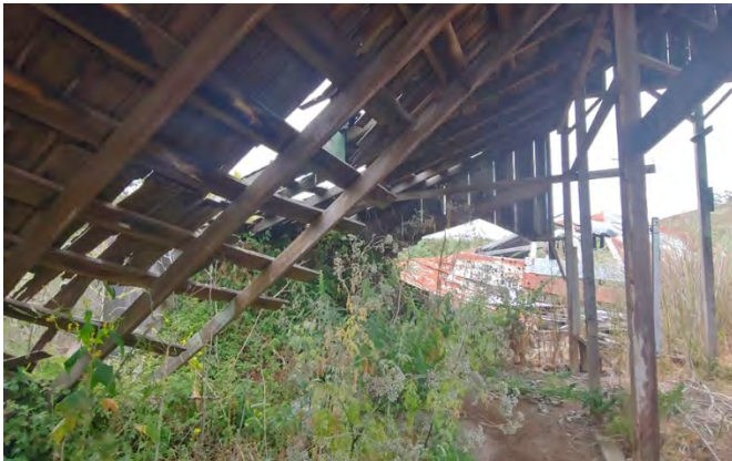
Photo 10: Crib on north side of barn interior, view facing east. Unknown collapsed building in the background.
