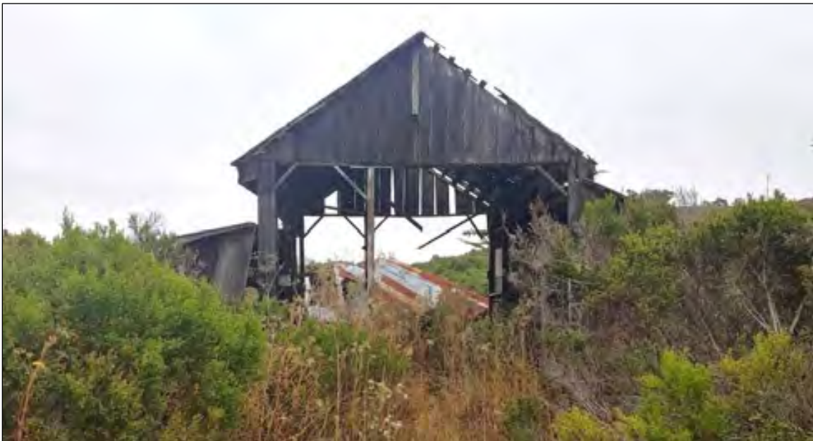
Figure 5-5 West elevation of the barn, view facing east. View obscured by vegetation.
