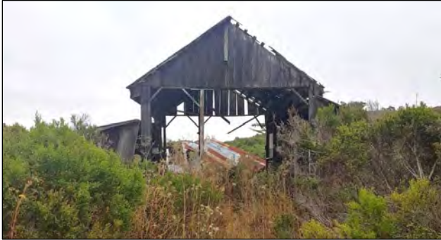
Photo 8: West elevation of the barn, view facing east. View obscured by vegetation.
