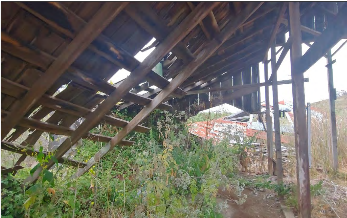
Figure 5-7 Crib on north side of barn interior, view facing east. Unknown collapsed building in the background.
